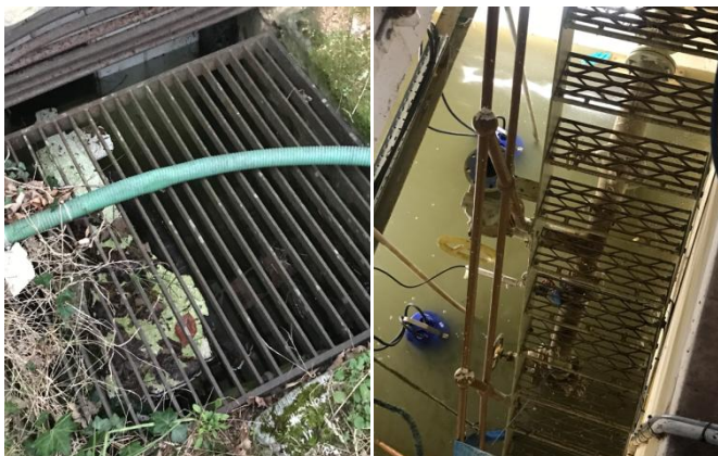
Anglian water pump station 5ft under water, sewage overflowing onto farm premises.
